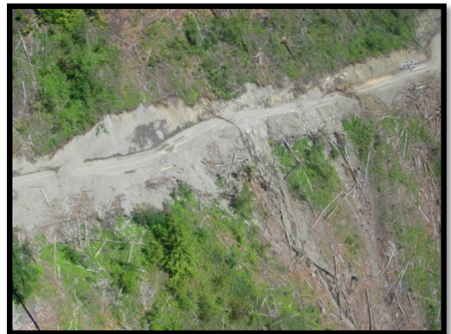
Engineered road construction causing erosion and sedimentation into a fish bearing stream.
