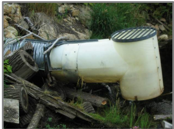
Figure 11. A water line is visible on the beaver proof add-on indicating it was controlling the lake level.
