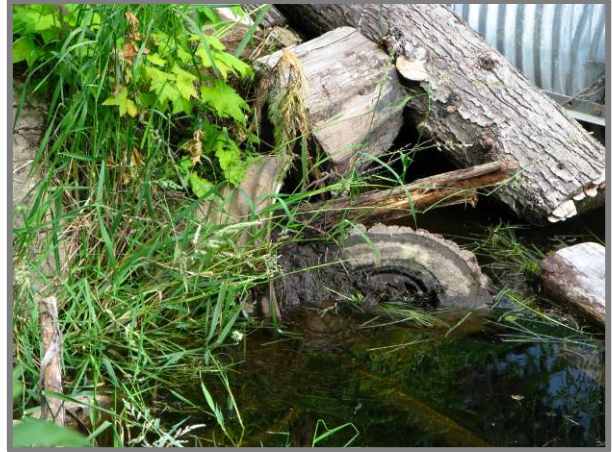
Figure 16. July 12, 2013 – Close-up of the lower culvert inlet described as "mostly blocked" by the complainant. The upper beaver proof culvert is visible in the top right.
