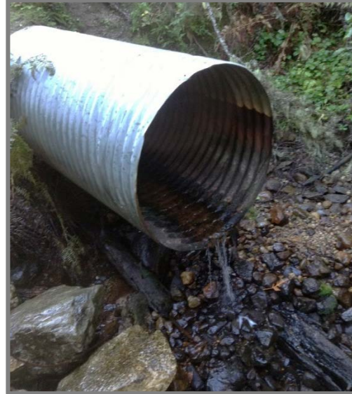
Figure 19. September 17, 2013 – The original culvert outlet is passing only a small amount of water indicating that it is almost completely blocked. Rust marks show how high the flow was in the past.
