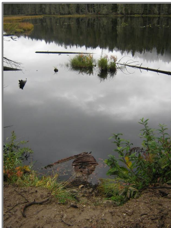
Figure 7. October 4, 2007 – The culvert inlet is damaged and almost completely submerged. A second culvert with a beaver proof add-on was installed five days later.
