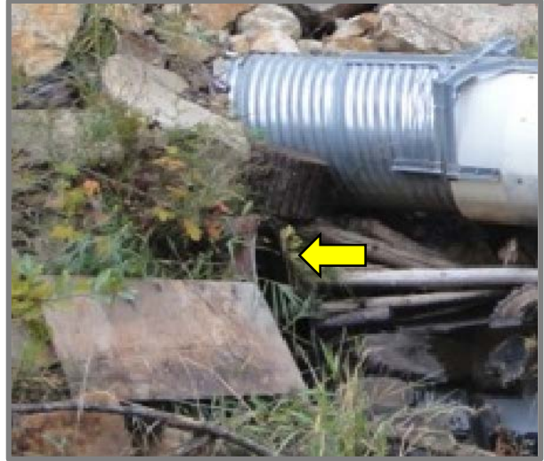
Figure 9. Close up of the previous photo. The arrow points to the lower culvert inlet.
