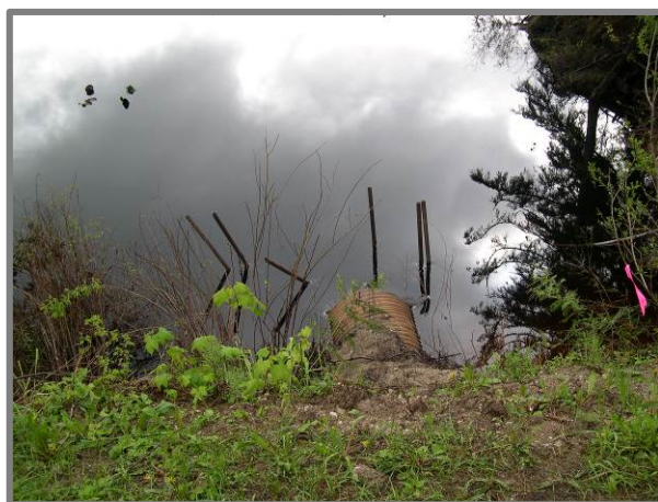
Figure 5. May 31, 2004 – The culvert is once again functional. The metal pipes of the debris catch are intended to prevent debris from entering the culvert.
