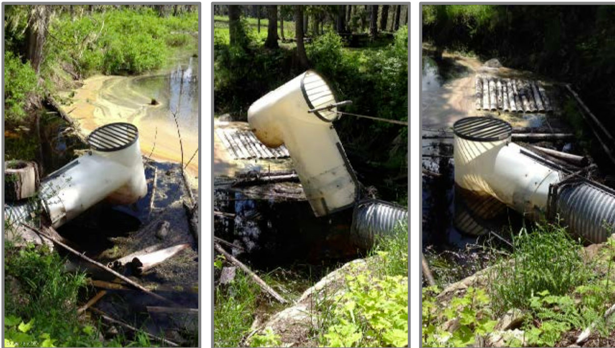
Figures 12, 13, 14. June 13, 2013 – Ministry inspection photos. (Left) The beaver proof add-on held aloft by debris. (Middle) Staff pulled up the add-on to clean it out. (Right) The add-on was put back in place.
