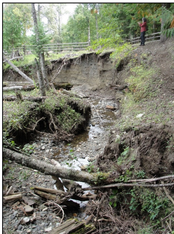
Figure 3. Evidence of stream bank erosion was observed on most sections of Bonneau Creek that flow through the complainant's private land.
