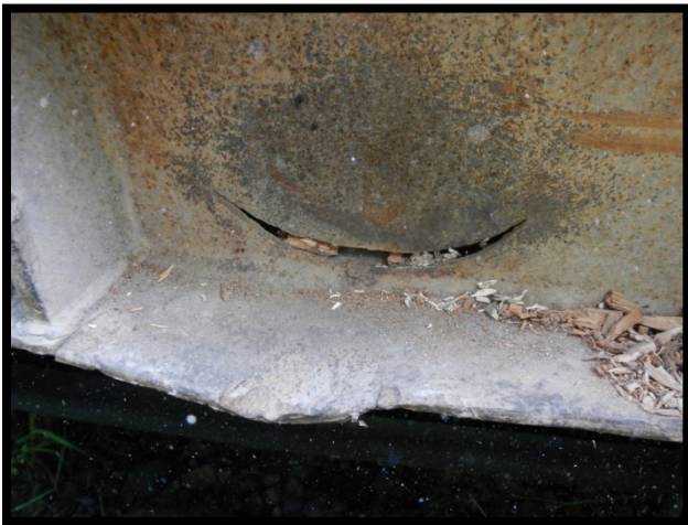
Structural fatigue evident on portable bridge by bearing stiffener.
