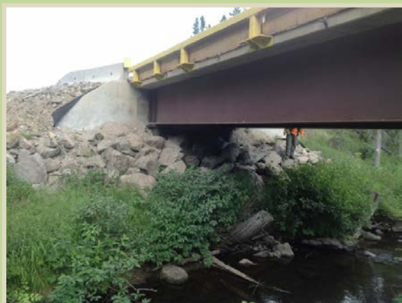
This bridge abutment is well armored and placed outside of the stream channel to prevent scour.
