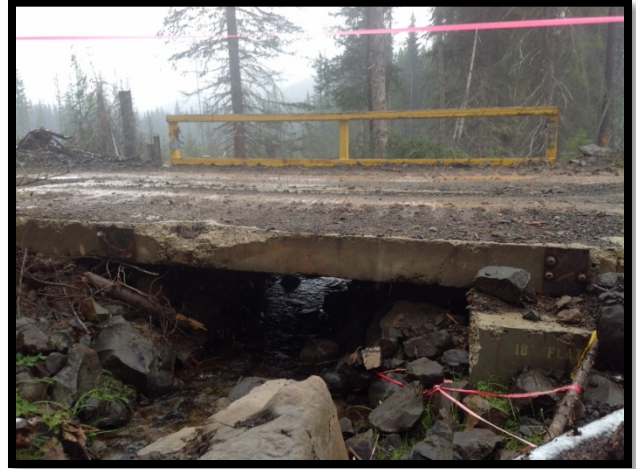
Concrete slab bridge missing guard rail.
