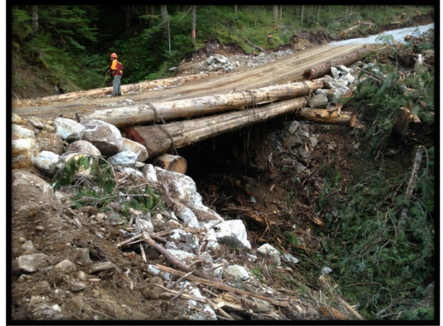
Unprotected and disturbed banks.
