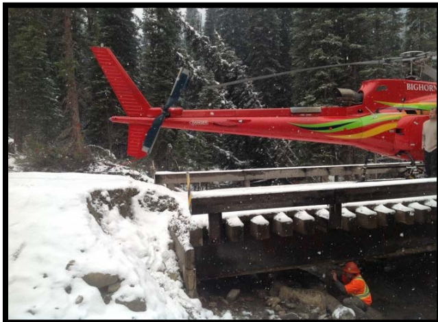
Abutment erosion. The abutment (log sills) washed away and the bridge settled 75 cm below the road surface.
