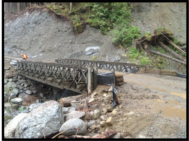
There was no professional assurance that this portable superstructure is safe for re-use at this site.
