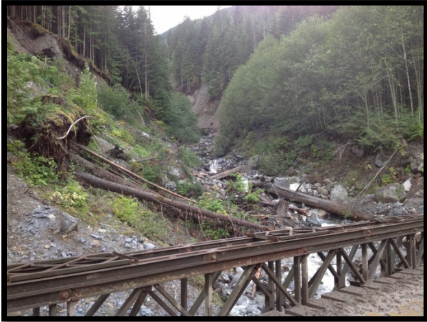
Unstable channel above bridge with no consideration of channel geomorphology or anticipated flows. No information provided by licensee.
