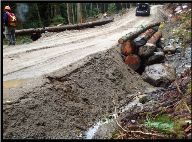
Unstable and erodible fill in the approach is a safety issue and also contributes sediment to the stream.
