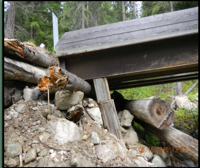
A poorly constructed bridge identified in a Forest Practices Board audit.
