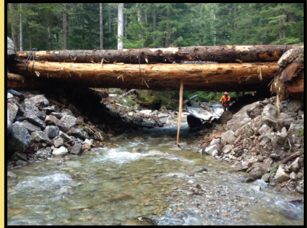
This bridge is too short for the stream and the rip-rap is constricting the channel. Natural surface drainage is not maintained.
