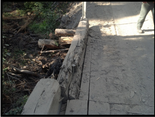
Deck panels differ in width. Narrow panel shows damage from a vehicle.
