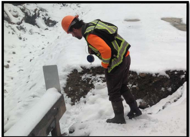
A close-up view of the settling due to abutment erosion.
