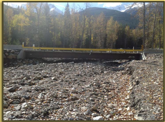
Insufficient clearance after a storm event due to aggradation (deposited sediment and gravel).
