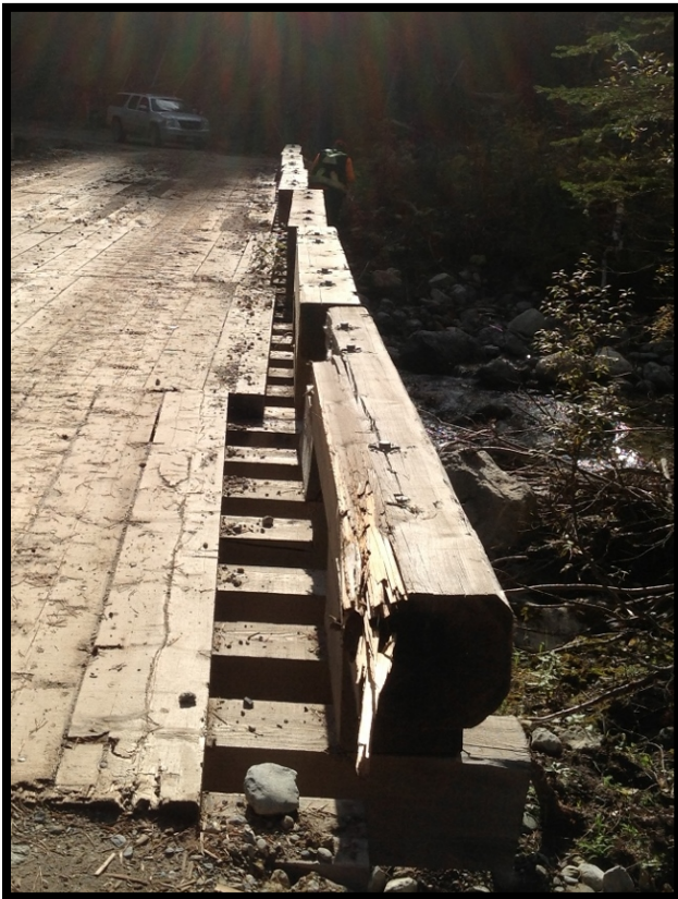
Deck panels have shifted because they are not attached to the girders.
