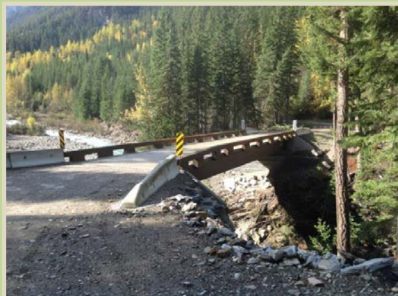
This bridge has concrete "no-posts" on the approaches to direct traffic onto the bridge deck.
