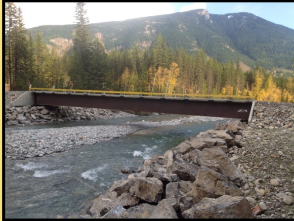
This bridge spans the channel and the rip-rap does not encroach on the stream. Natural surface drainage is maintained.
