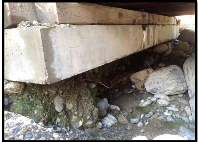
Close-up of same bridge. Extensive scour under the foundation after a major storm event.
