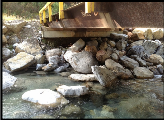
Abutment erosion resulting from inadequate foundations installed well above creek scour depth, constructed within stream channel. An improperly supported substructure could ultimately result in structural failure of the bridge.
