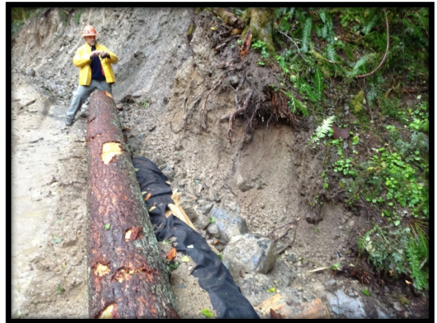
Poor sediment control. Sediment from the cutbank in the background can wash into the stream affecting water quality.
