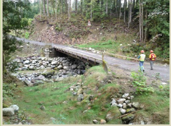
This bridge has safe approaches and the channel and abutments are protected with rip-rap.
